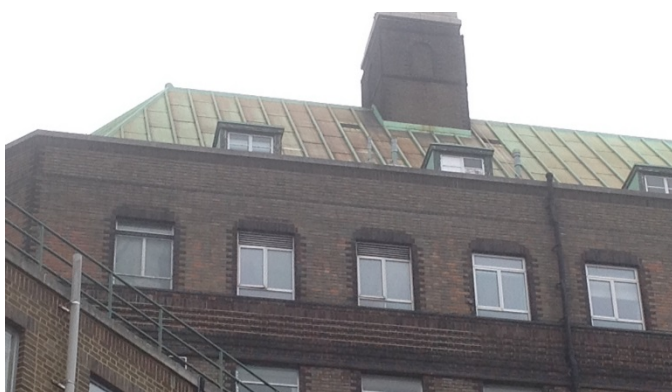
Figure 8: discoloured existing copper roof
